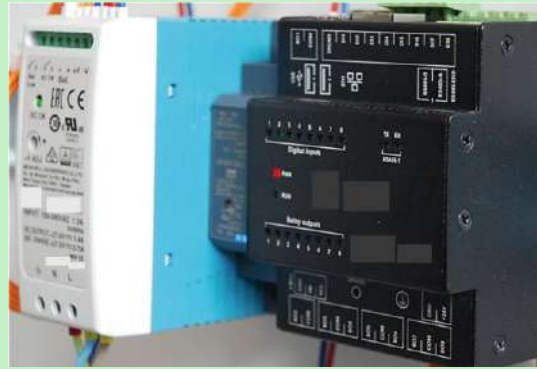
Battery Power supply for PLC
